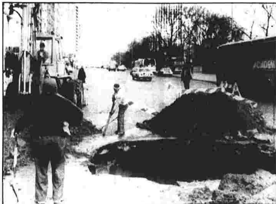
POCK-MARKED PARK — New York City water department workers tend to a 15-foot hole in the pavement off Central Park South in Manhattan Friday. The hole was caused by a broken water main, which disrupted subway service and caused major inconveniences on the biggest shopping day of the year.
